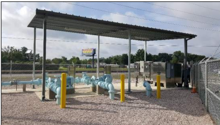
Figure 8 View to south of booster pumps at Water Plant No. 5
